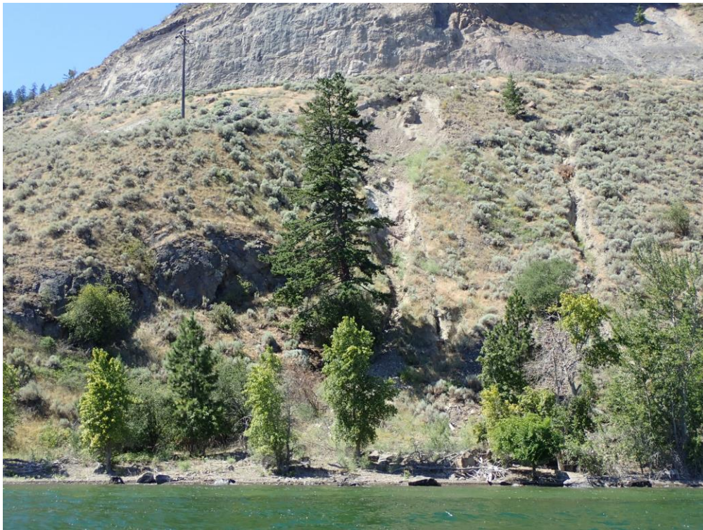
A washout below a Highway 97 drainage culvert on Crown land, Okanagan Lake, July 2019. The vegetated buffer at the lakeshore captures some sediment.
